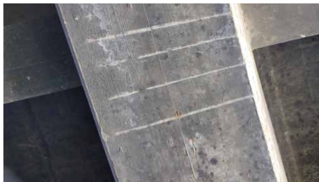
Figure 5: Confirmation of 0.1-mm cracks (PCT girder)
