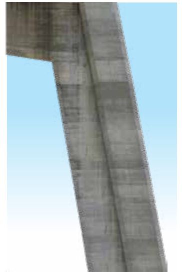
Figure 6: Crack path documentation of a bridge tower.
