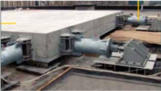
Figure 8: Tuned Mass Dampers installation at Bucharest Romania by GERB [6]
