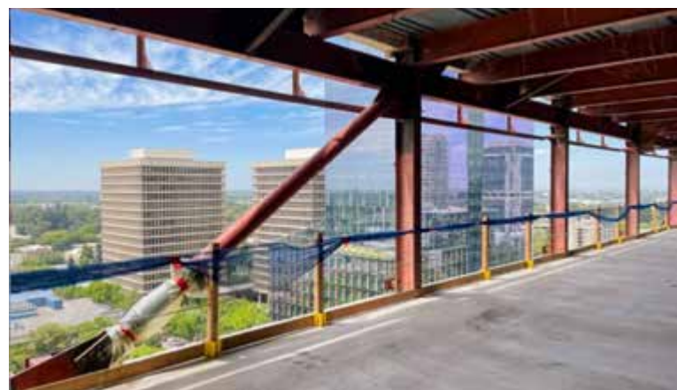
Figure 2: 17-story State of California Resources Building built in 1962, with steel truss moment frames, 128 nos. FVDs installed to retrofit by Taylor Devices [17]
