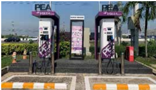
(a) charging stations
