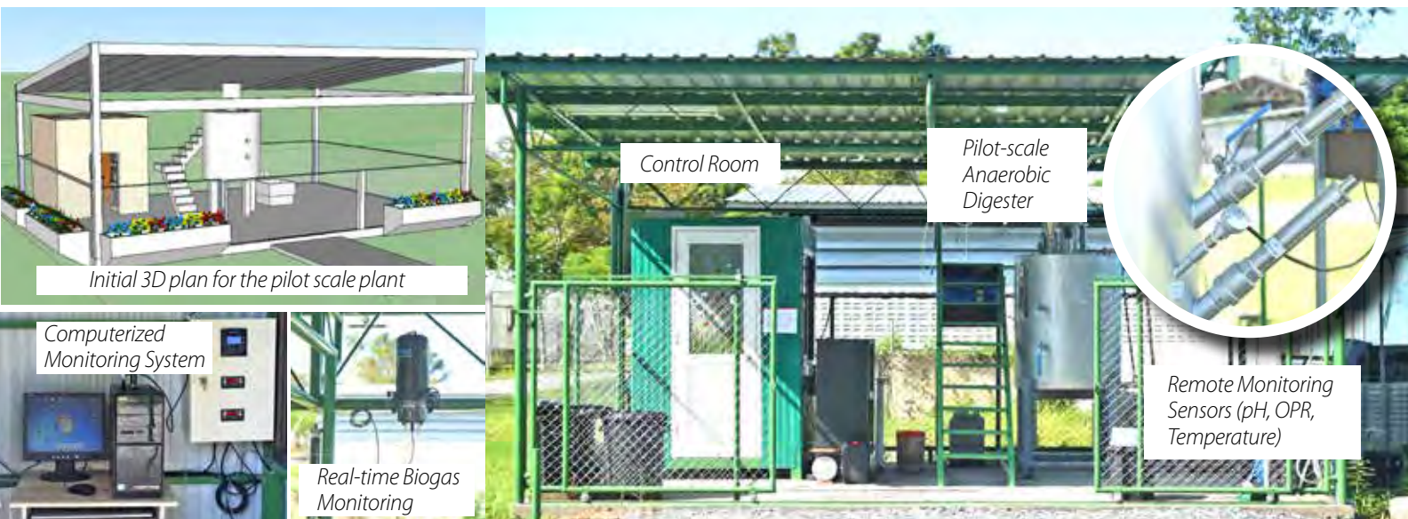
Figure 4: IoT based Decentralized Anaerobic Digestion
