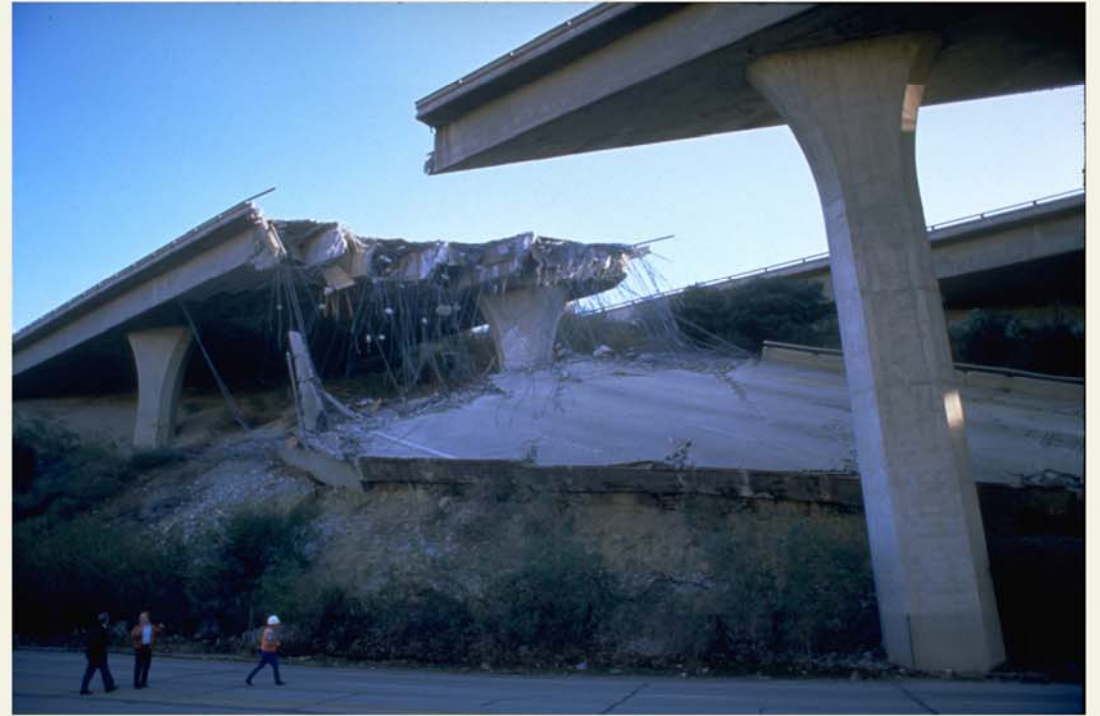
Damaged portion of the Golden State Freeway at Gavin Canyon.
