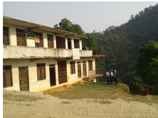
Figure2: Typical load bearing masonry school building which experienced moderate shaking in Kavrepalanchowk, it became unsafe due to major cracks in unreinforced partition walls.
