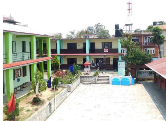
Figure12: A school building in Kathmandu shows different response. The building at the back, load bearing masonry was moderately damaged in the earthquake and the building at the left, load bearing masonry, retrofitted with concrete jacket was undamaged and was available immediately for restarting classes after earthquake.
