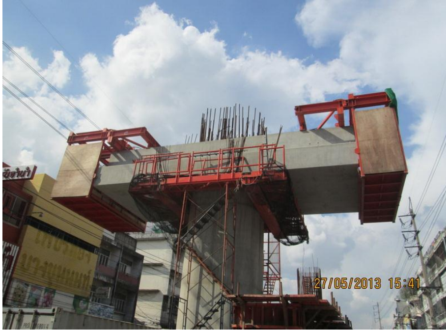
Installation of Crossbeam Interface Segment (IF) at BN16/3 (Concourse Level) Bang Khun Non Station – Zone 5
