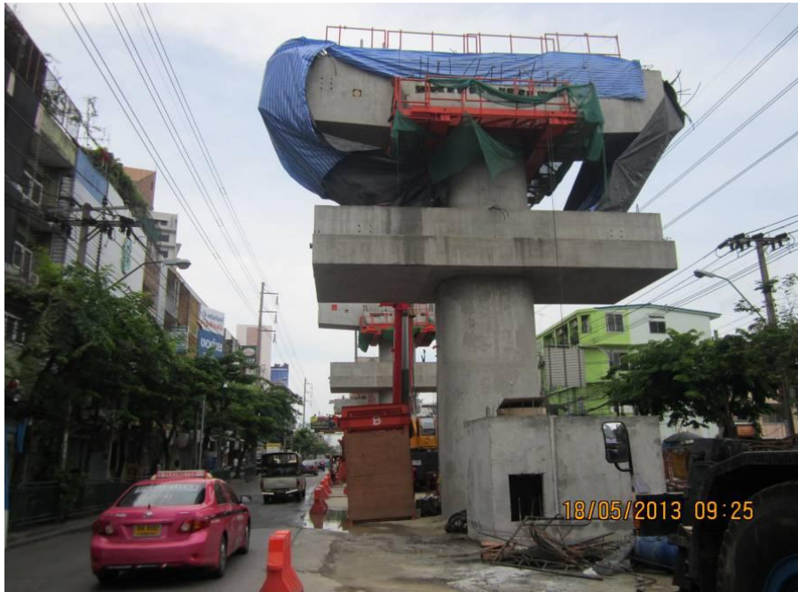
Installation of Crossbeam Segment at BN18/3 (Platform Level) Charn Sanit Wong Station – Zone 5
