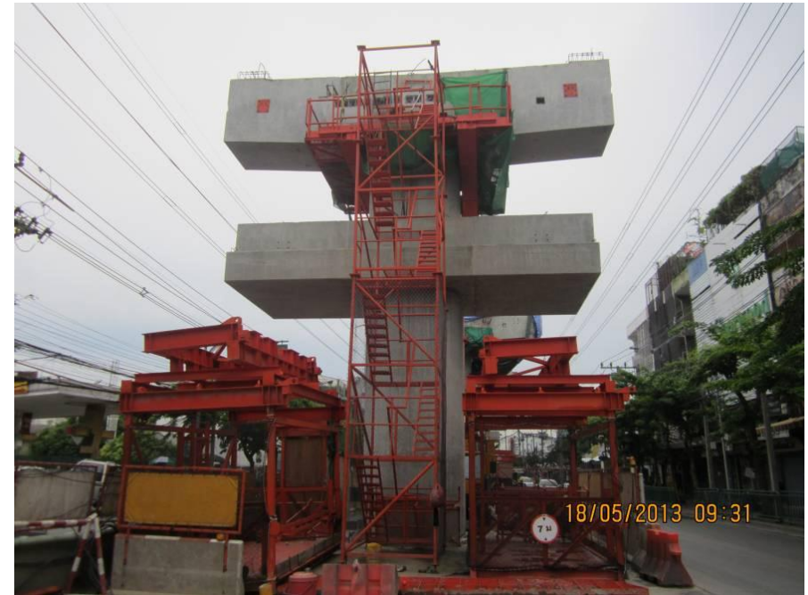
Installation of Crossbeam Segment at BN18/4 (Platform Level) Charn Sanit Wong Station – Zone 5
