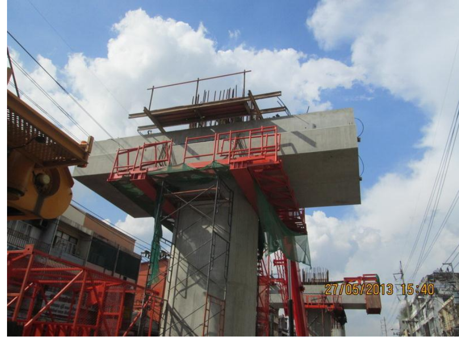
Installation of Crossbeam Interface Segment (IF) at BN16/4 (Concourse Level) Bang Khun Non Station – Zone 5
